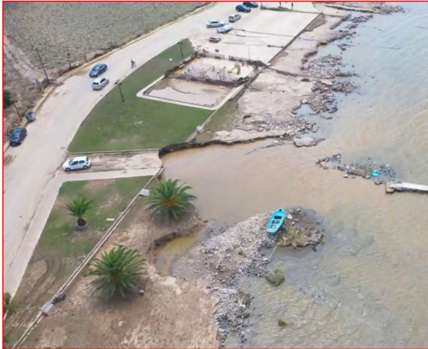
Erosion of coastal infrastructure at Mpourtzi
