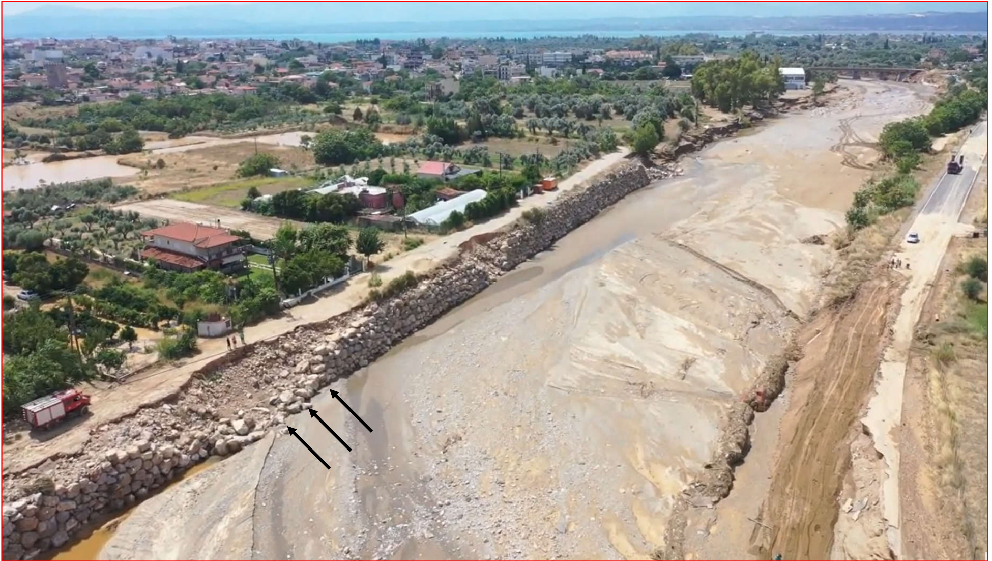
View of eroded bank protection works at the left bank of Lilas R. (looking downstream).
