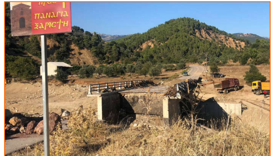
COLLAPSE OF BRIDGE NEAR MISTROS
