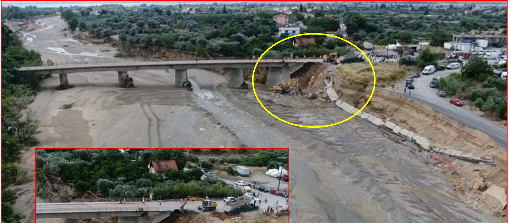
UAV pictures of damages in Vassiliko Bridge (looking downstream)
