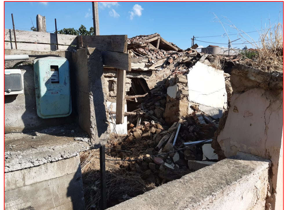
Impacts on stone-built houses (Lilas R. floodplain) Complete collapse
